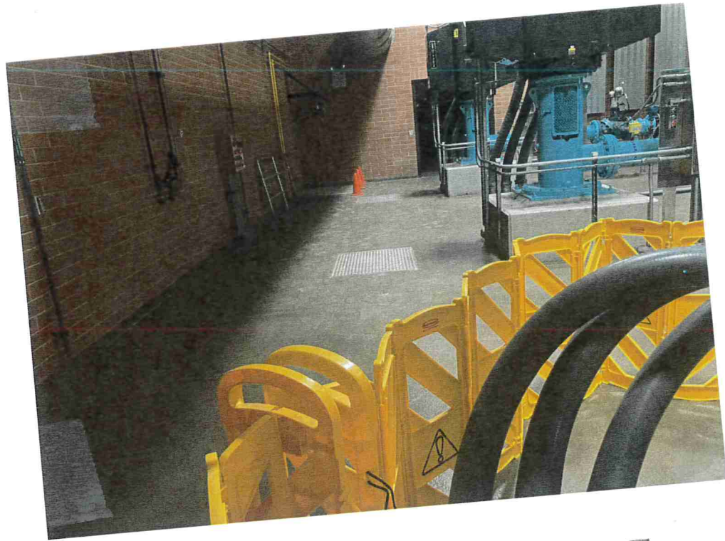
① REPLACE DIAMOND PLATE WITH FRP GRATING
