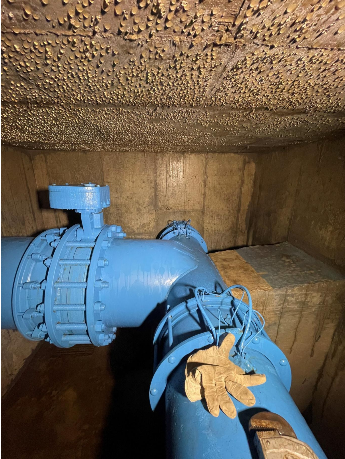
9365 S 2286 E Vault
