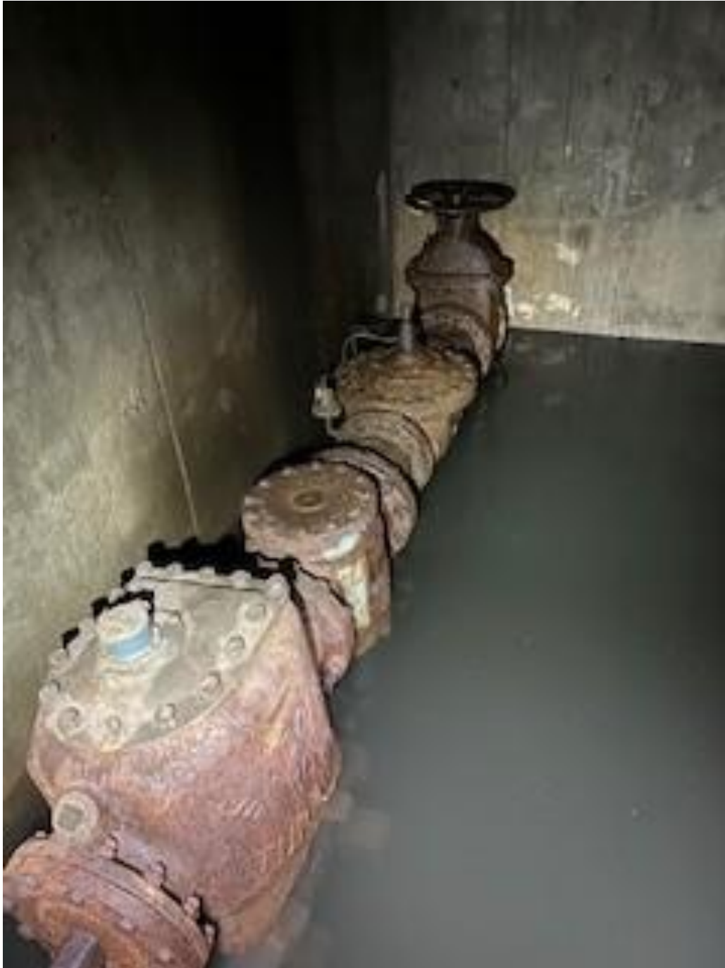
11400 S 1300 E Vault
