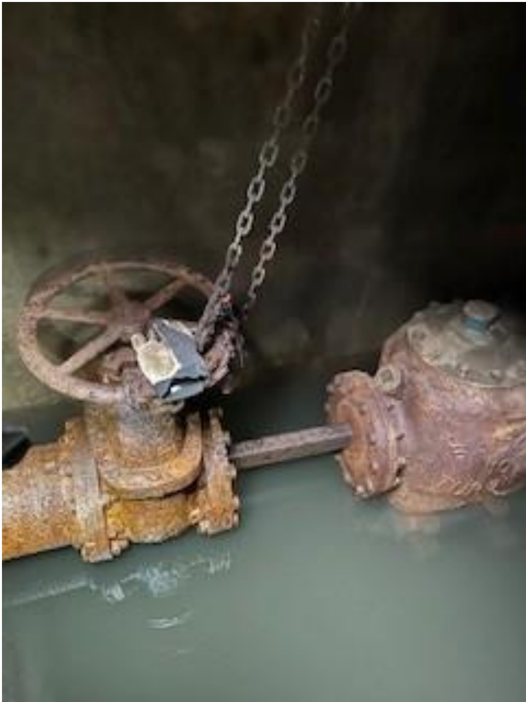
11400 S 1300 E Vault
