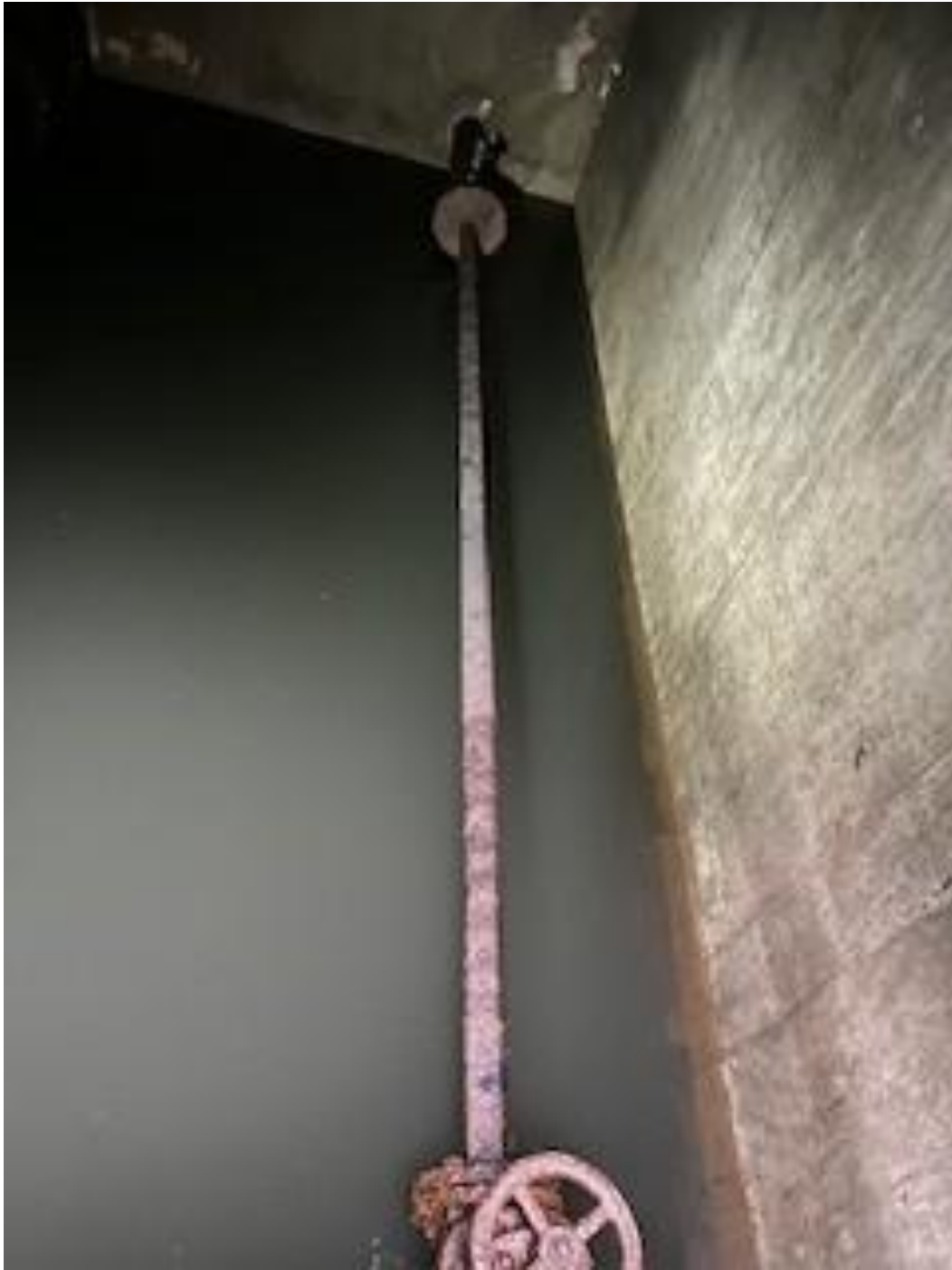
11400 S 1300 E Vault
