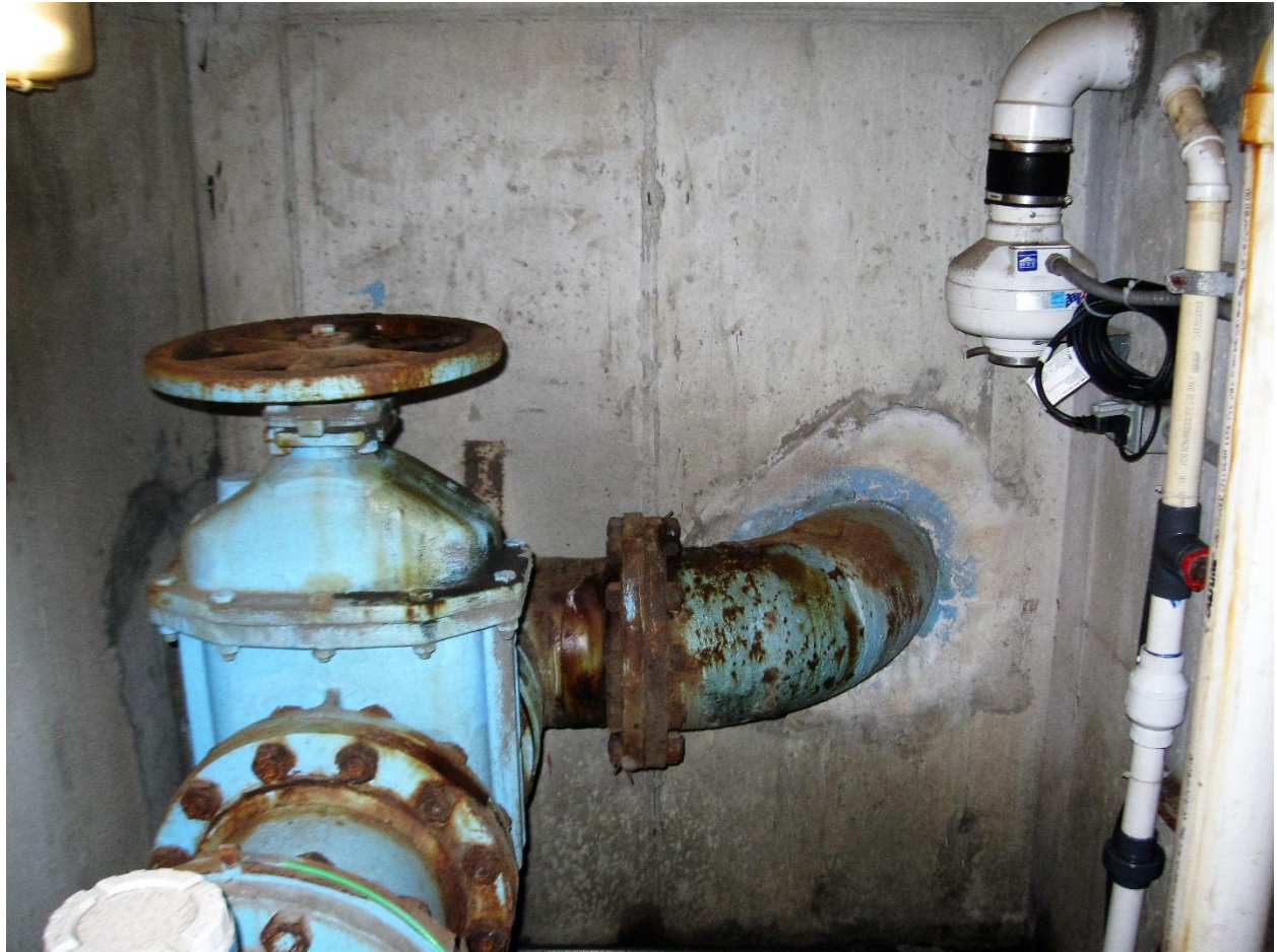
7500 S 175 W Vault
