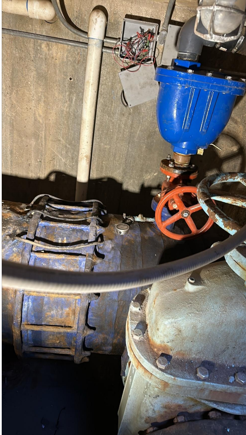
11400 S 1700 E Vault
