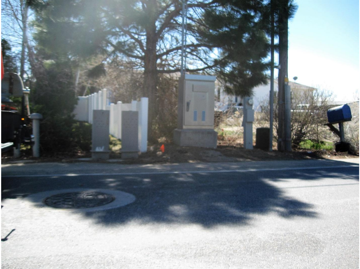
11400 S 1700 E Vault
