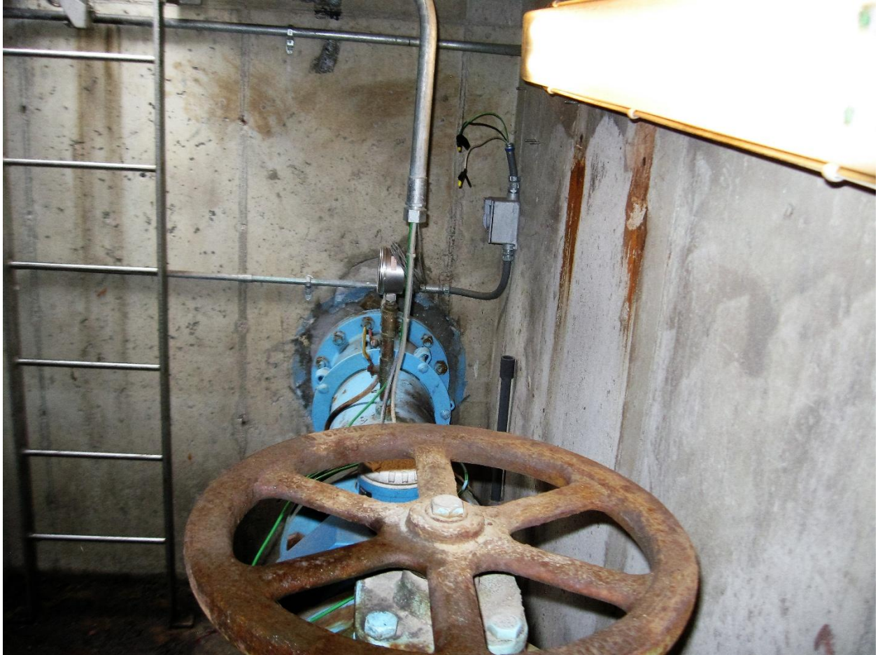
7500 S 175 W Vault
