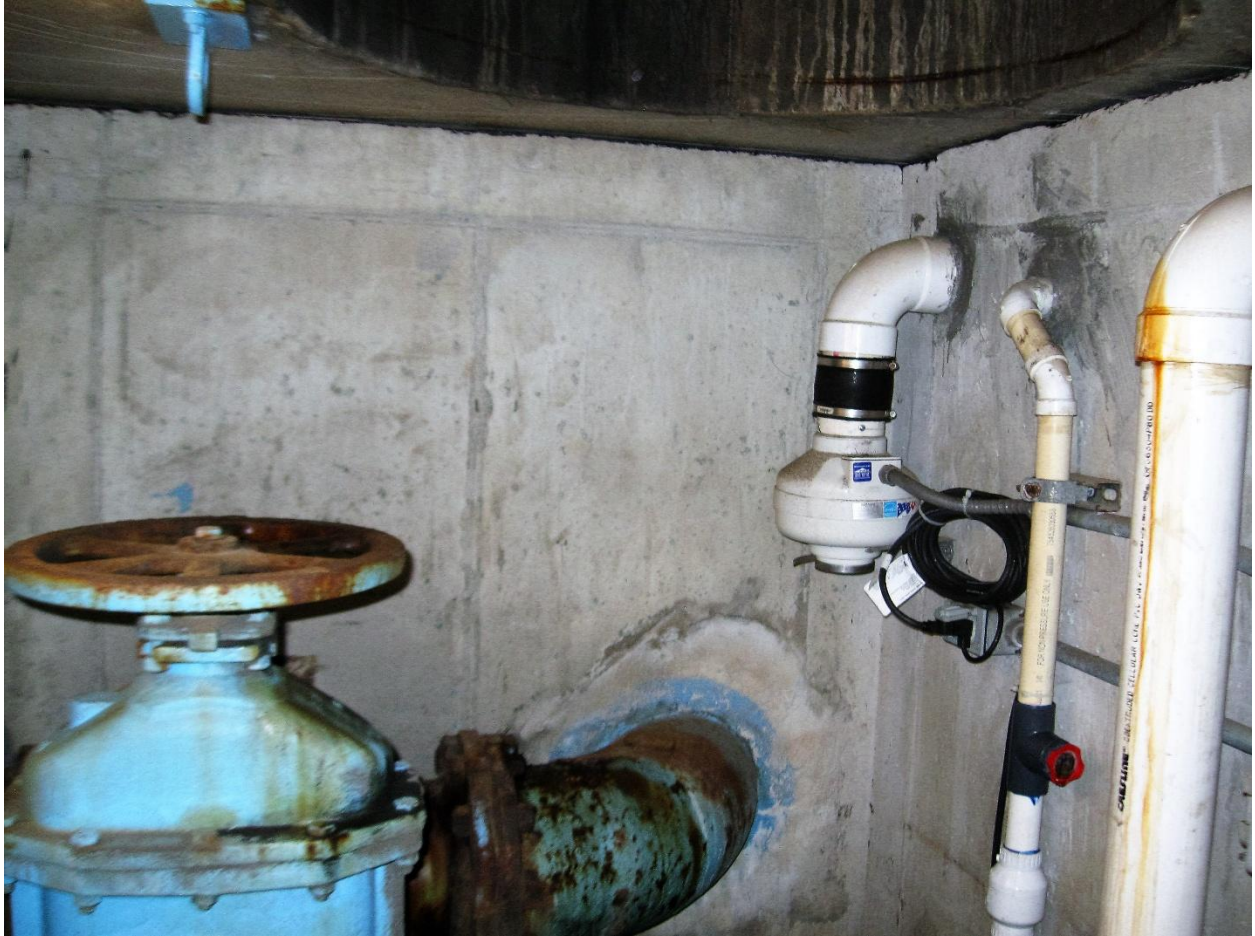
7500 S 175 W Vault
