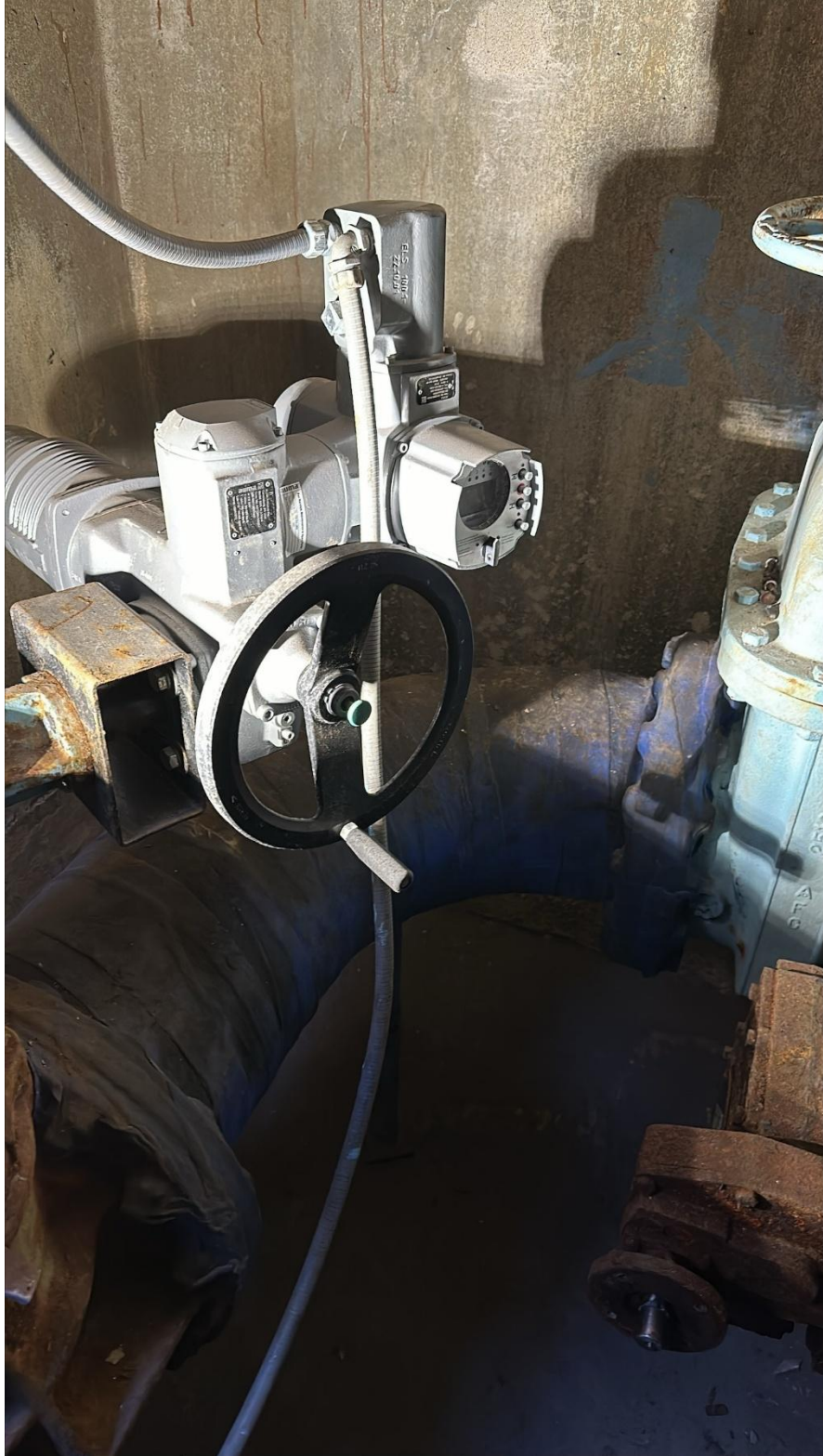
11400 S 1700 E Vault
