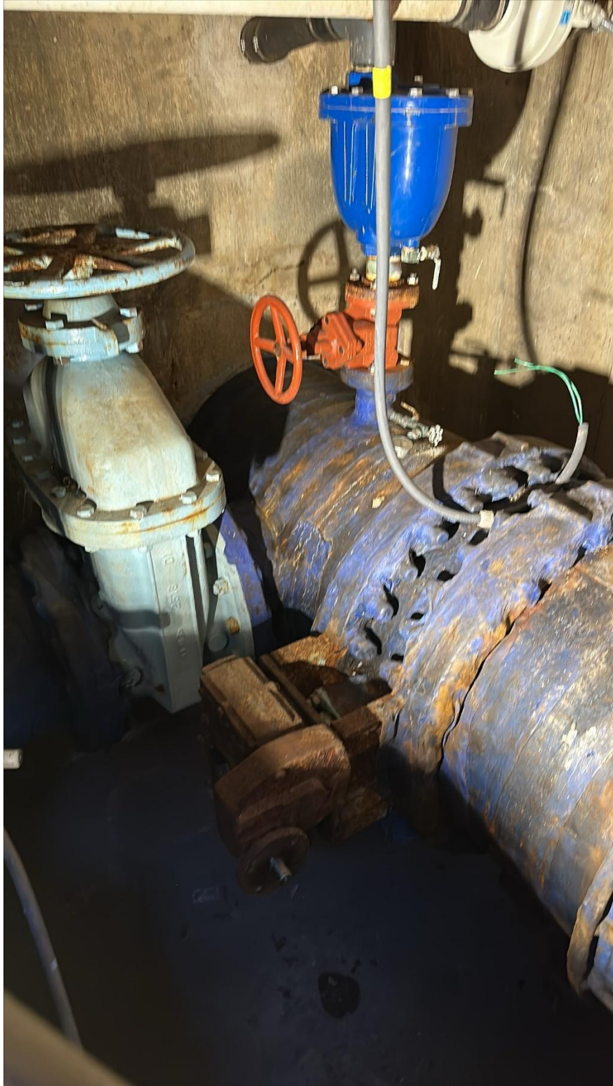
11400 S 1700 E Vault
