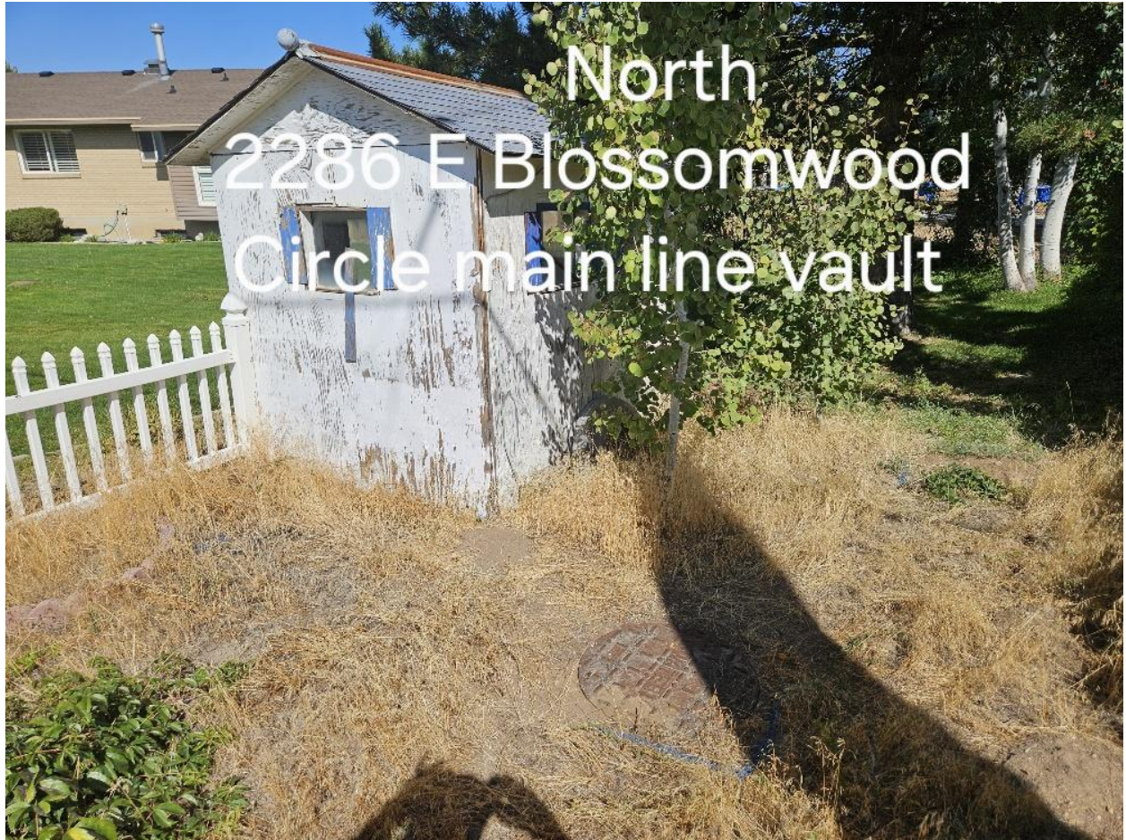
9365 S 2286 E Vault
