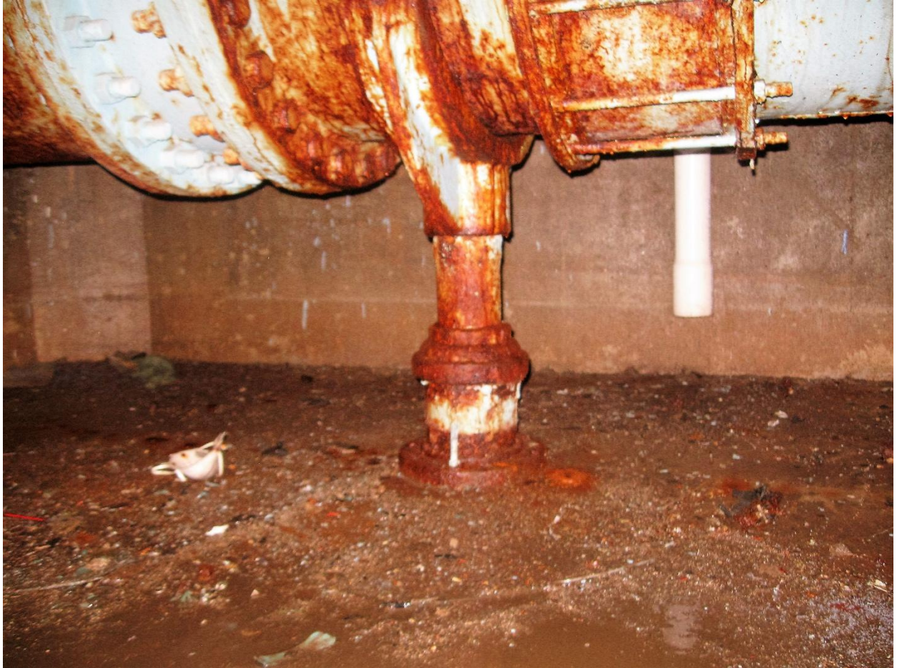
11400 S 1700 E Vault
