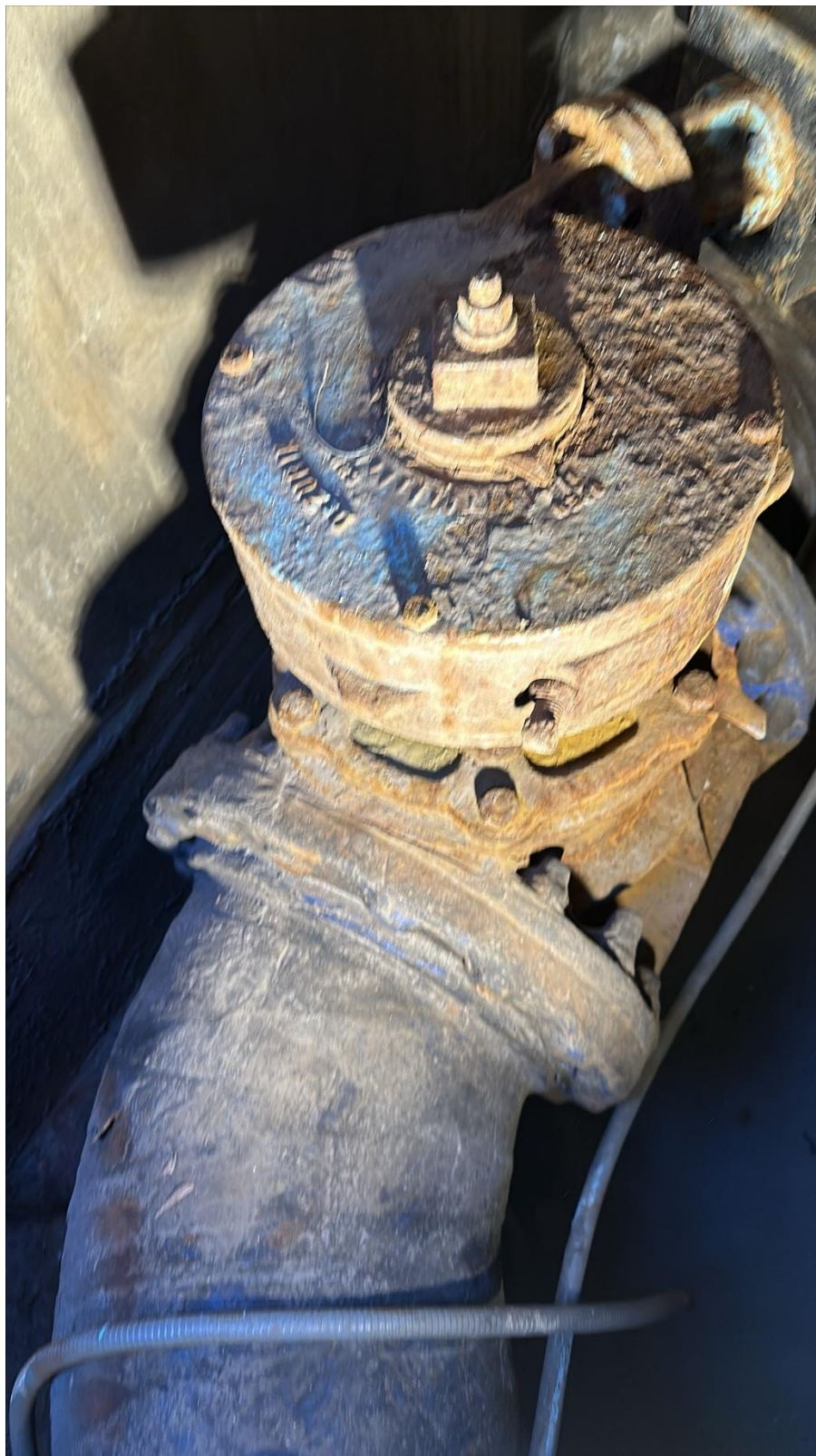
11400 S 1700 E Vault
