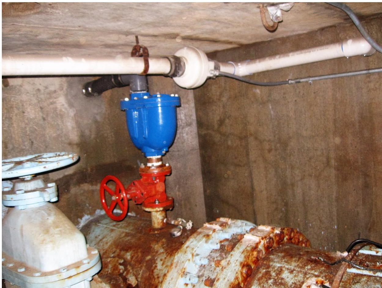
11400 S 1700 E Vault
