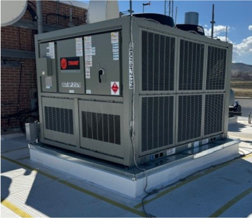
New rooftop chiller
