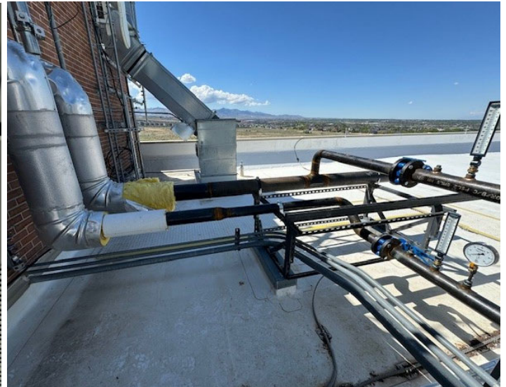
Piping routed into the building
