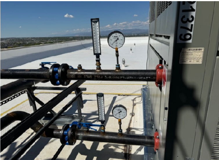
New piping and gauges
