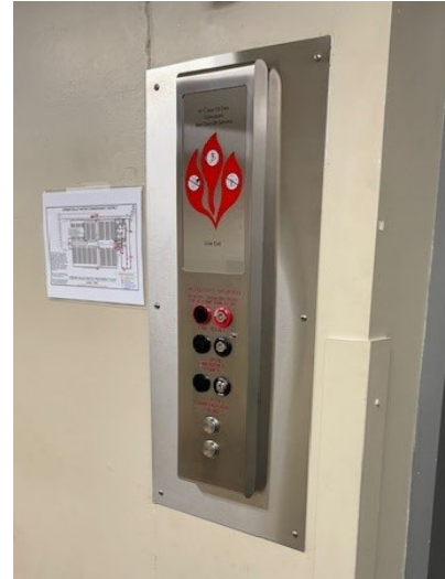
New controls and faceplate
