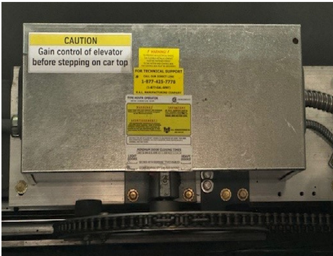
Elevator electronic controls
