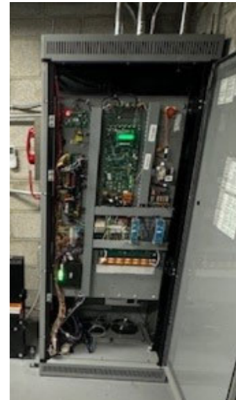
New electronics cabinet
