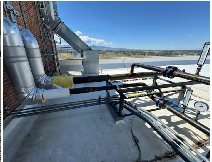
Piping routed into the building
