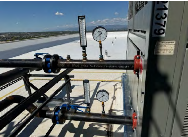
New piping and gauges
