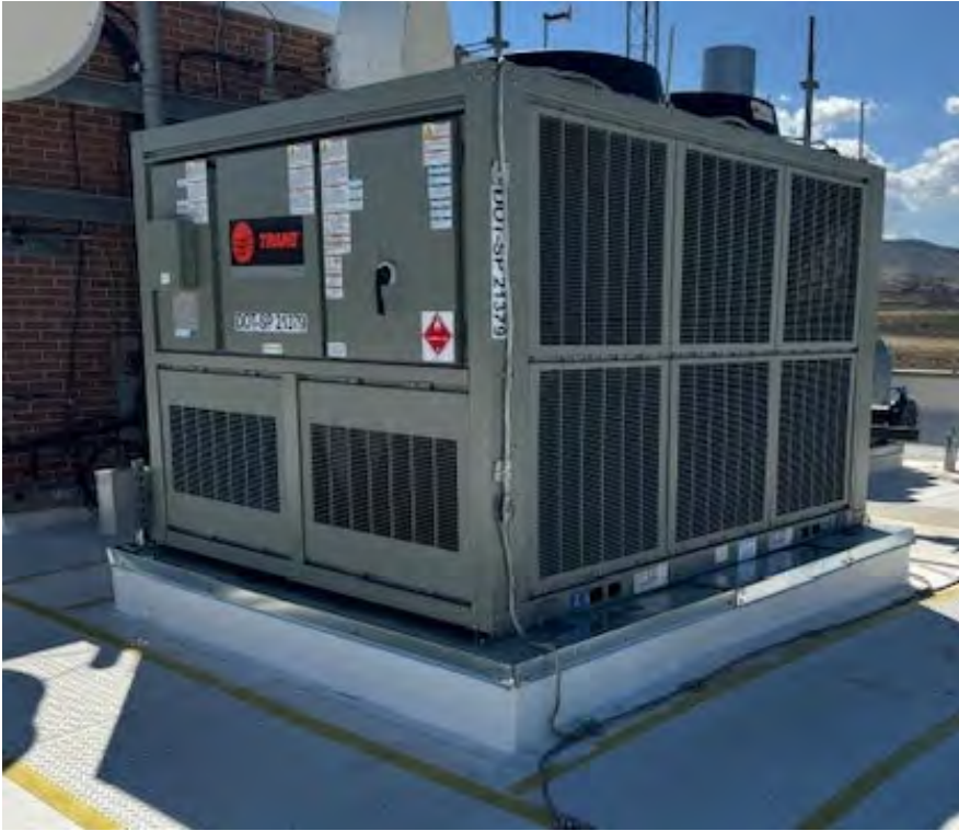
New rooftop chiller
