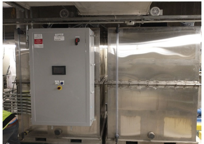
New Bulk Tanks and Control Panel
