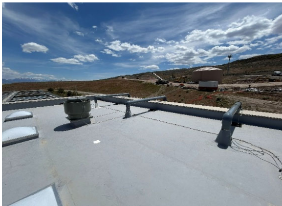
Tank vent extensions and new exhaust fans on Chlorine Dioxide Building
