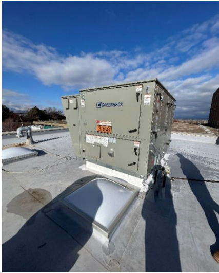
New make up air unit on Chlorine Dioxide Building
