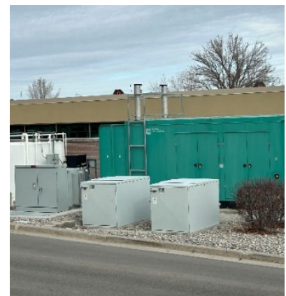
New generator exhaust stacks
