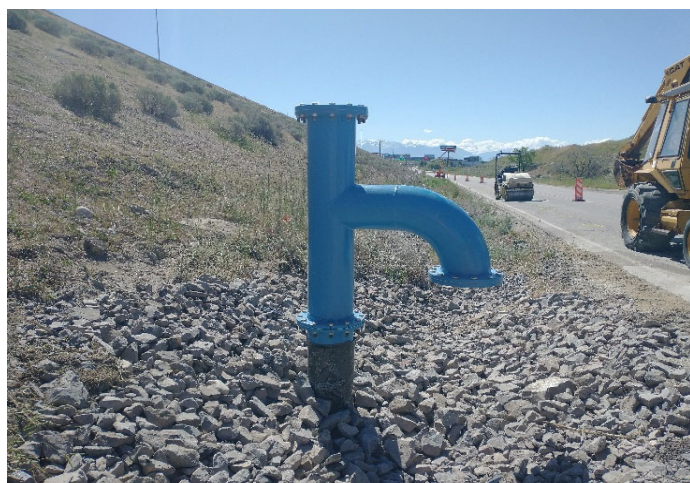
New Blowoff in UDOT canal
