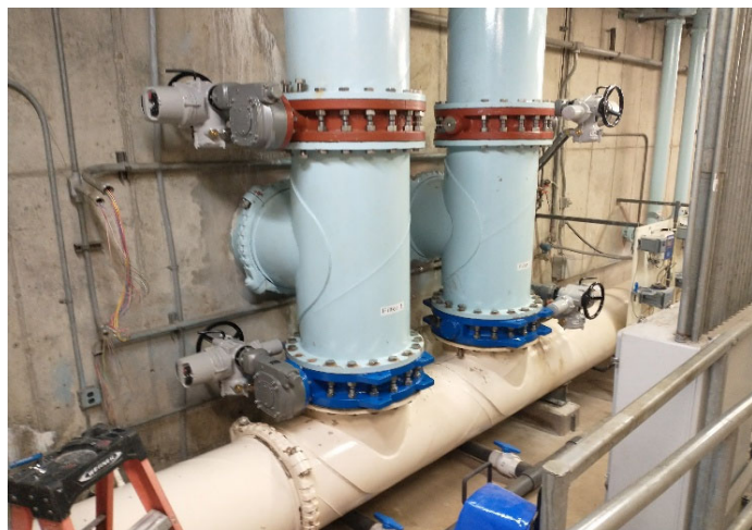
New Valves and actuators in filter gallery
