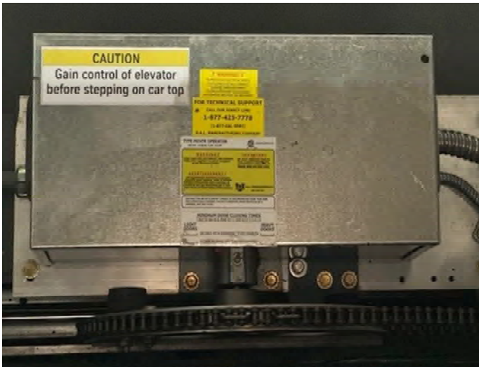
Elevator electronic controls
