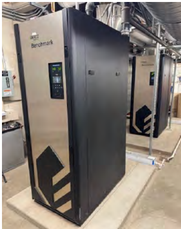
Boilers north view
