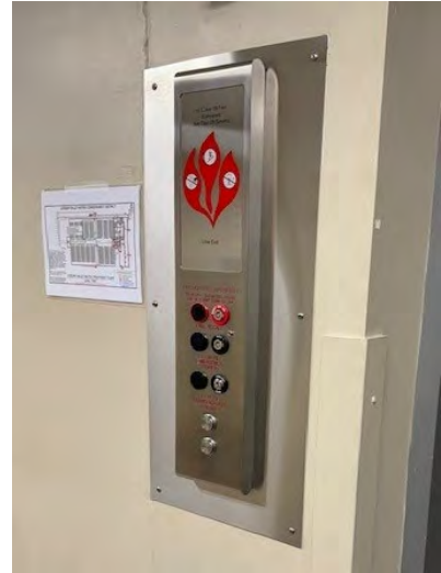
New controls and faceplate
