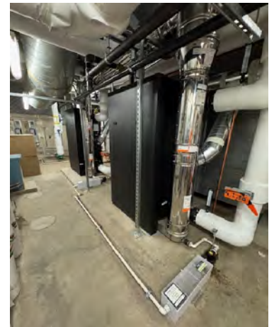
Boilers and exhausts east view
