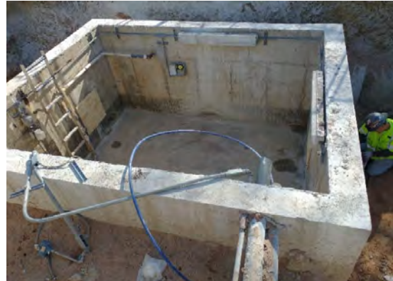
Vault with piping and lid removed
