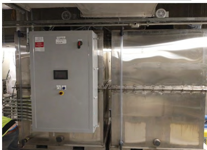
New bulk tanks and control panel
