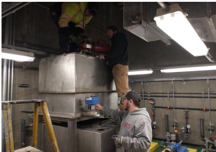
Original polymer bulk tanks
