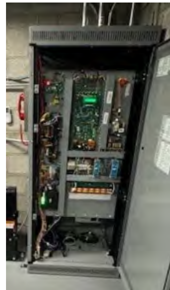
New electronics cabinet
