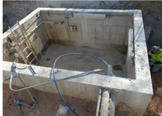
Vault with piping and lid removed
