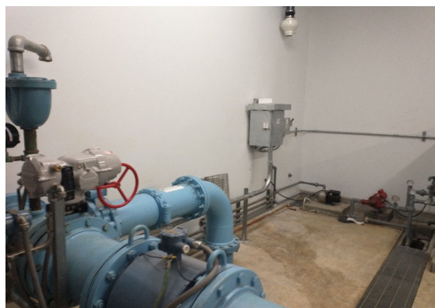
New rectifier for well cathodic protection
