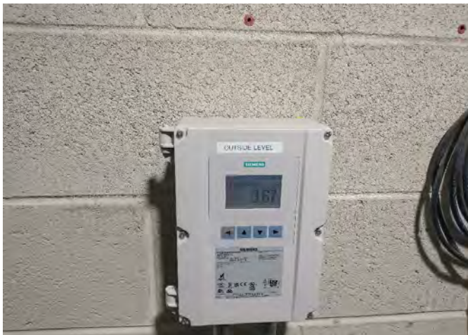
Level sensor display in the diversion structure
