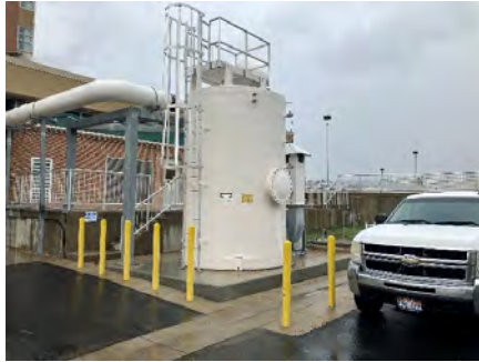
Chlorine Gas Safety Scrubber to be relocated as part of this project
