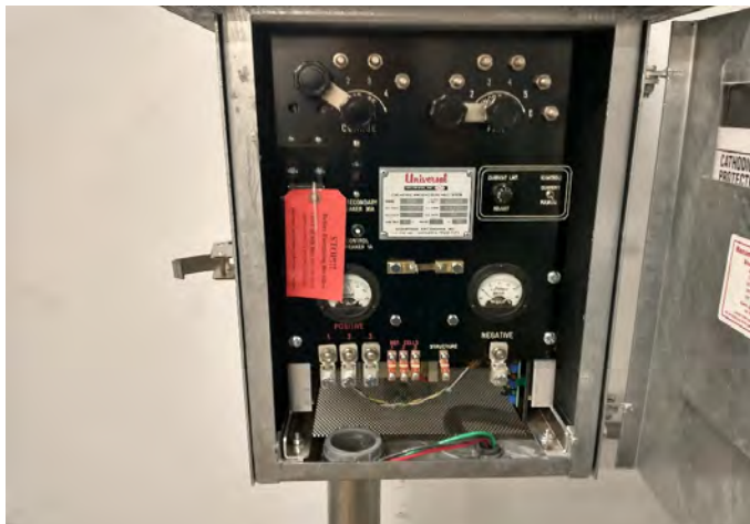
New well cathodic protection rectifier
