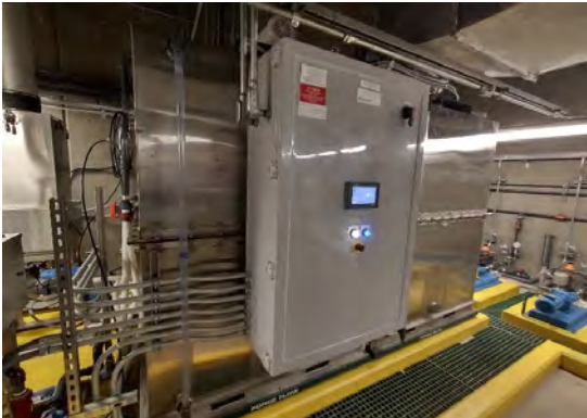
Control panel on side of tanks where new programming was added
