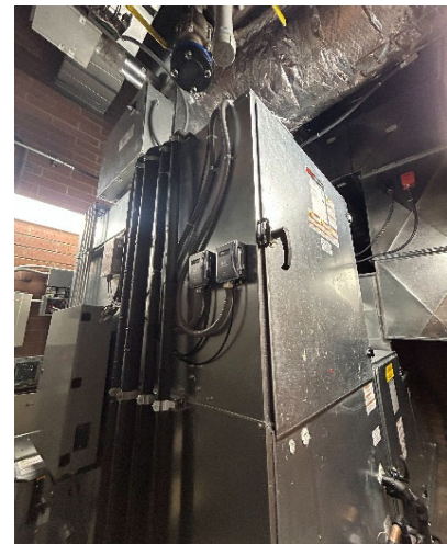
New air handling unit at SWGWTP
