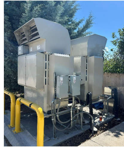
New heat pump unit and bollards at the Education Center
