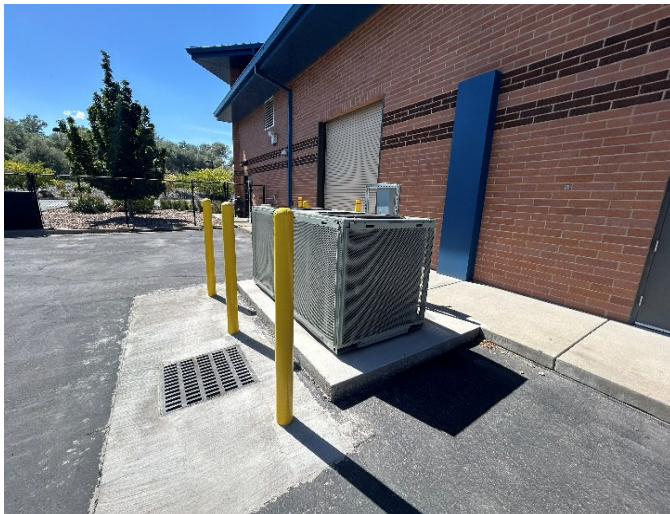
New air conditioning units at SWGWTP
