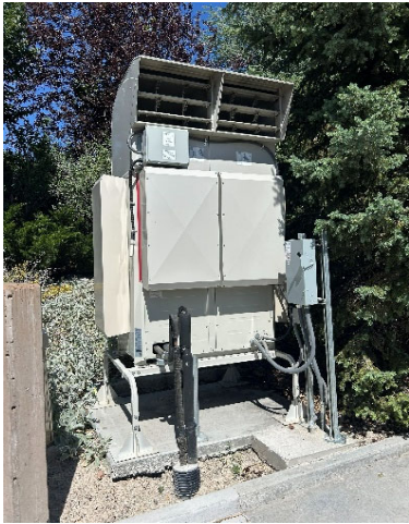
New heat pump unit at the Education Center
