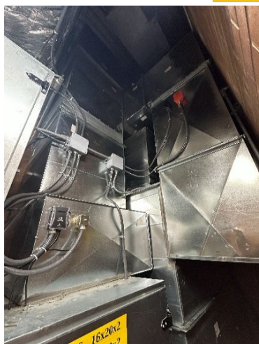
New air handling unit at SWGWTP
