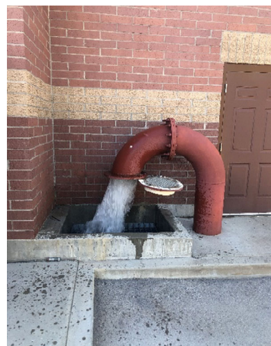
Pumping to waste during start-up
