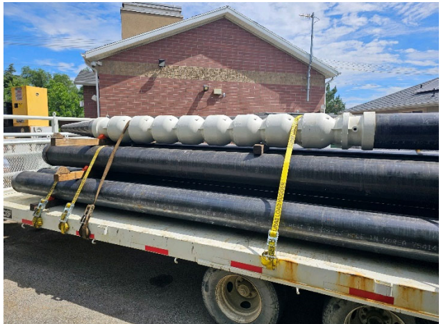
New pumping equipment
