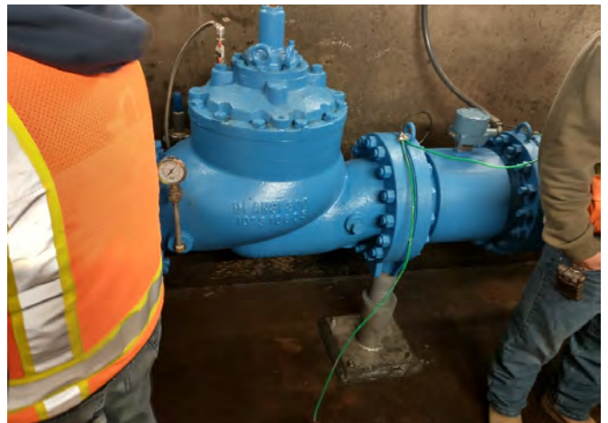
New PRV and flow meter installed in 700 East vault
