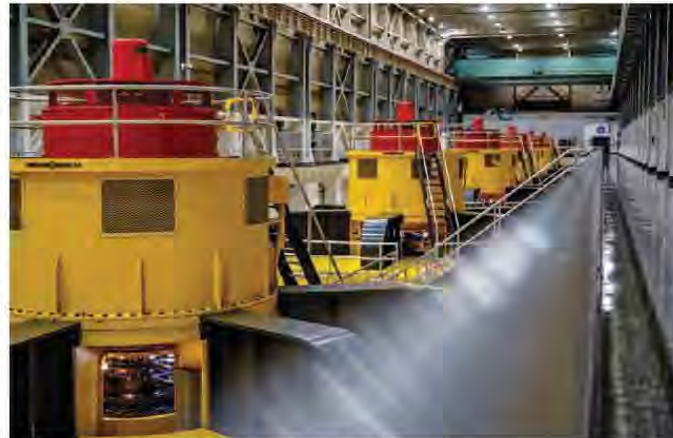
Some of the eight generators at Glen Canyon Dam in Page, Ariz.
