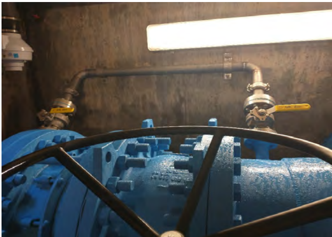
New valve and bypass installed in 110 East vault
