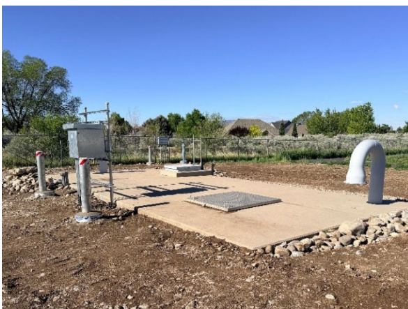
New rectifier and site restoration
