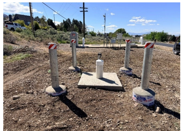
New anode well head
