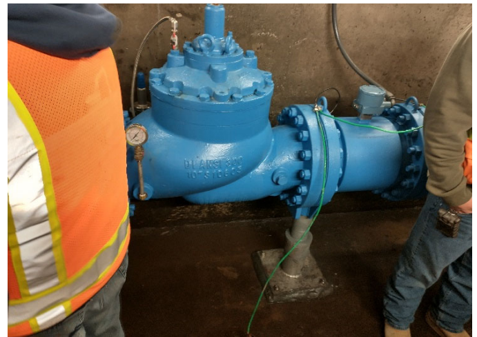
New meter and PRV at 700 E 11400 S
