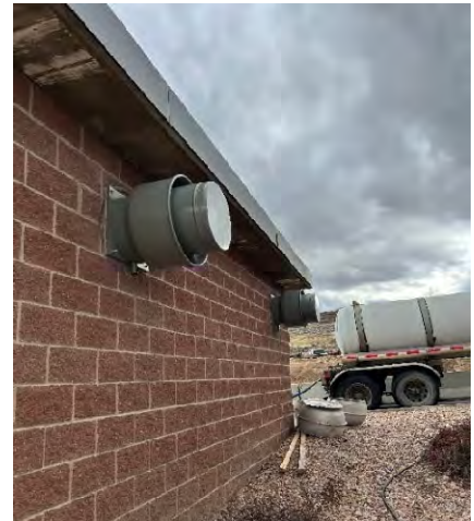
New exhaust fans on Alum Building
