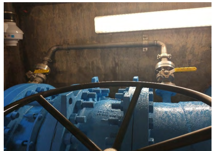
New mainline valve at 110 E 11400 S
