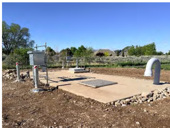
New rectifier and site restoration
