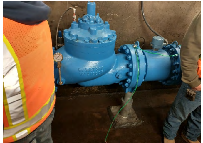
New meter and PRV at 700 E 11400 S
