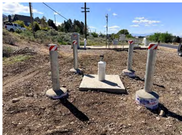
New anode well head
