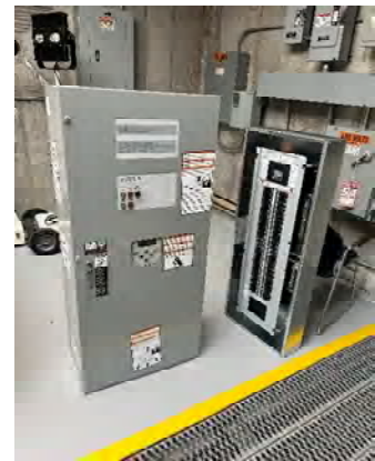
New automatic transfer switch and electrical panel
