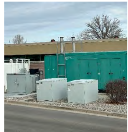
New generator exhaust stacks
